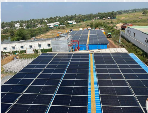
Venkateshwara Ice Factory, 143 KW. Repalle, Andhra Pradesh
