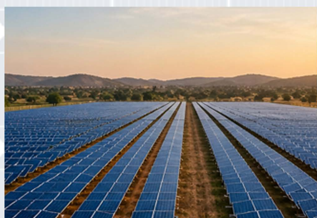
Surya Teja Power Projects, 2.4 MW Bhongir, Telangana
