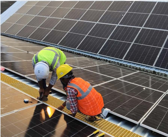
Ramya Spinning Mills, 600KW. Ganapavaram , Andhra Pradesh
