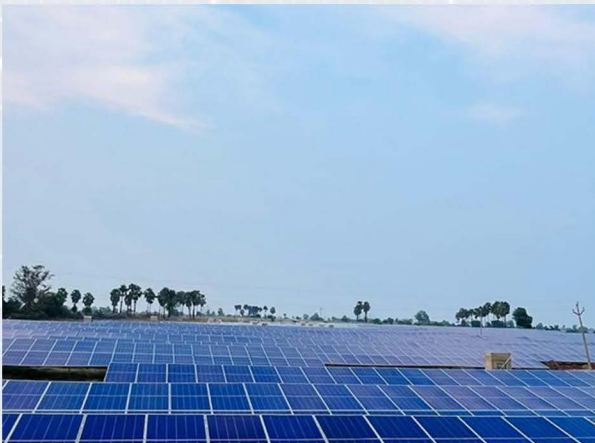
B.Vellamla Ground Mounted, 2.4 MW Narkatpally, Nalgonda, Telangana
