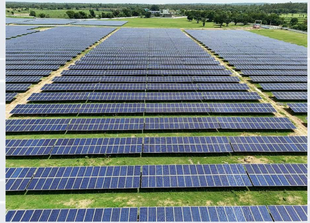
5 MW, Ground Mounted Plant. Parigi, Vikarabad district, Telangana
