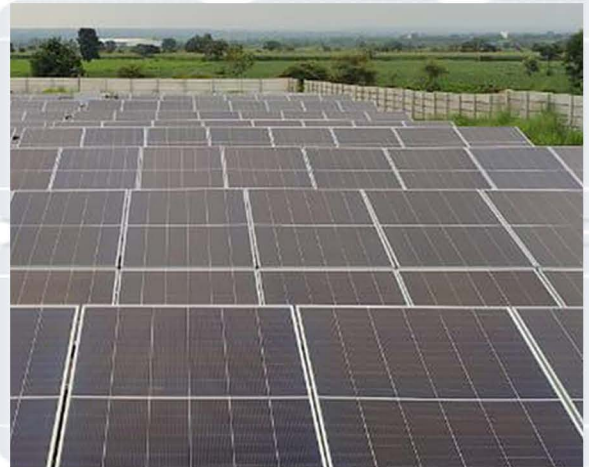
Alkimia Pharma - Chem Pvt.Ltd 600KW, Ground Mounted plant. Zaheerabad, Telangana
